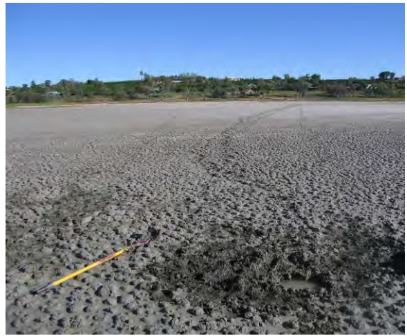
Figure 7-10. Photograph of Site 8, showing the site location near the centre of the wetland where the surface was cracking.
