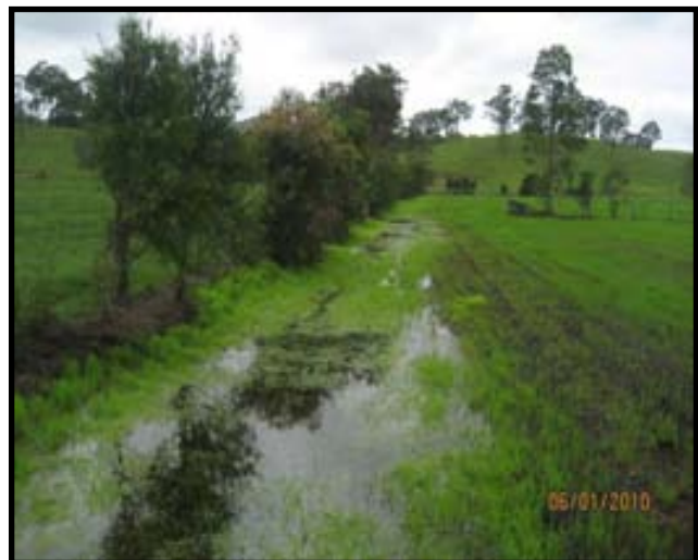
After: The drain has been limed, filled and remodelled to a 1km 600mm x 3500mm (average) channel displaying drain water pH 6.5 & good pastures growing
