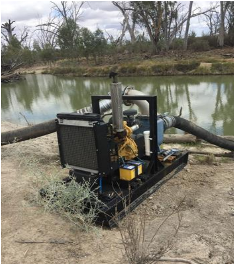
(a) Diesel pump with a capacity of 6 ML/Day
