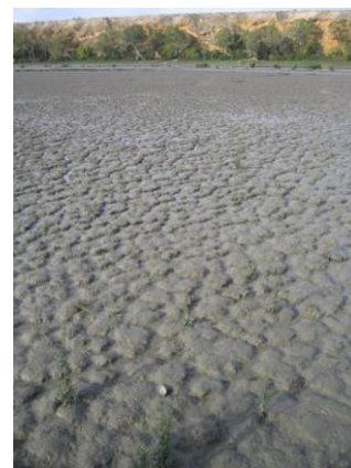
Figure 66-5. Photograph of site MLG4, showing the soft clay surface that had degraded and filled the soil cracks with the surface aggregates.
