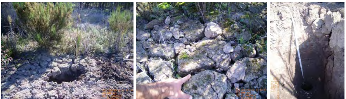
Figure 5 – Photographs of site 40383_3, showing the stream channel surface condition, cracking surface and the shallow soil profile of reddish brown, strong, silty clay loam and clay.
